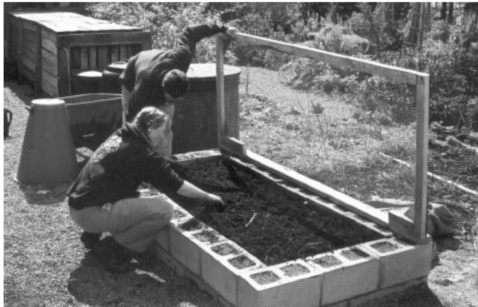
Above: Robin Gillmor and Chris Wells put the finishing touches on the worm pit.
